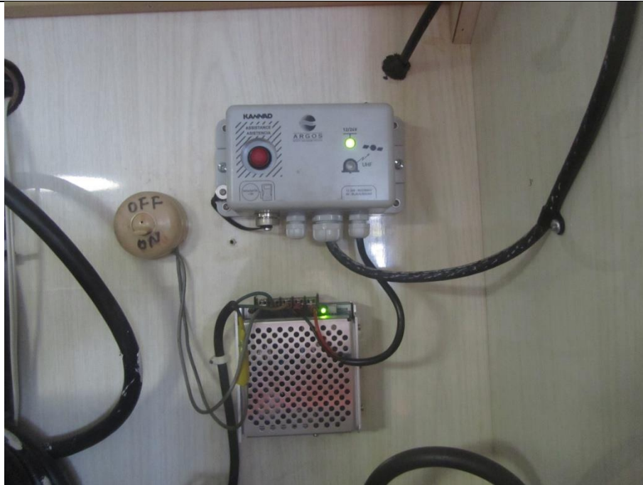
Figure 5 VMS of the xxx fitted with a power switch
